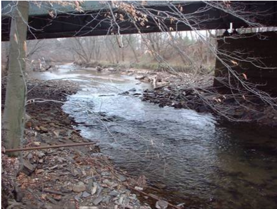
Bedrock riffle in dewatered impoundment under the PennDOT Huntingdon Pike Bridge, March, 2008
