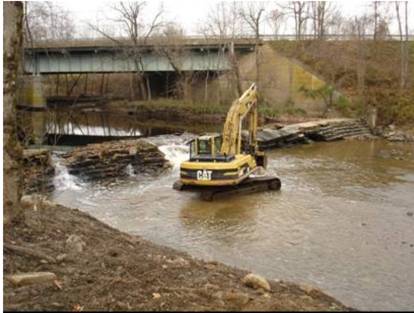
Removal of center dam course for impoundment dewatering and sediment control, December 2007
