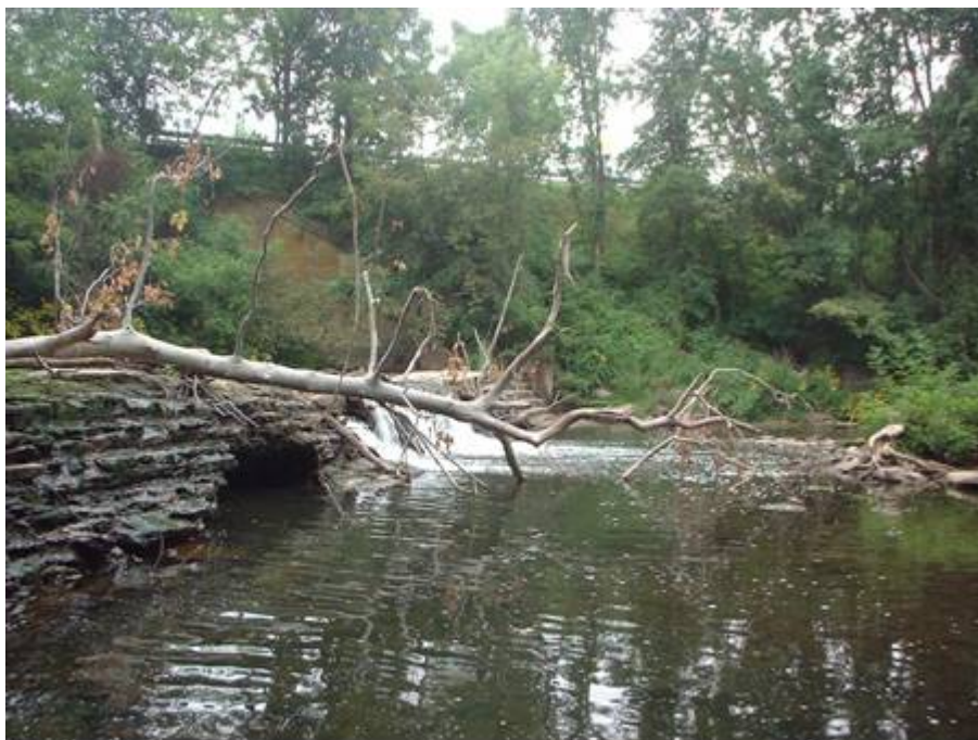
Plunge pool below slumped dam crest, September 2007
