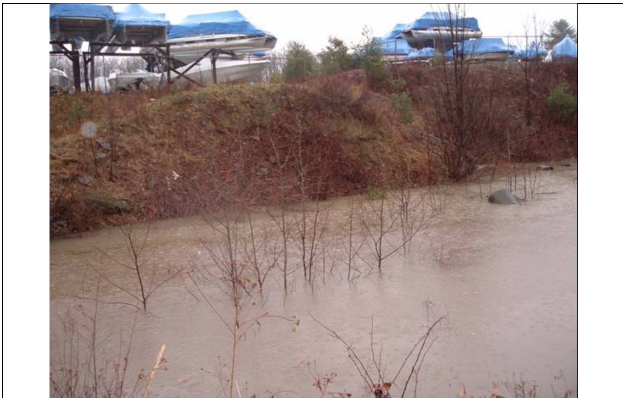
Poorly-functioning Detention Basin Adjacent To Bakker Marine Before BMPs Installed
