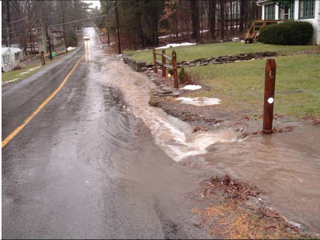
Roadside and Flooding during rain event before BMP installed
